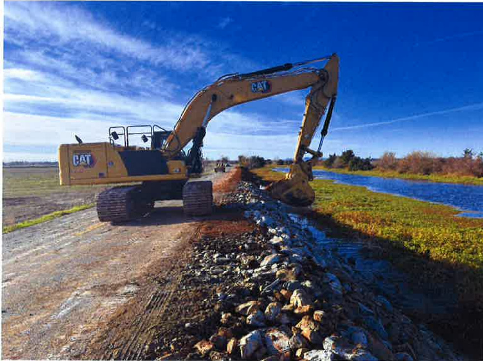
Placement of 18" minus riprap after re-establishing the waterside slope at the eastern site of repair.
