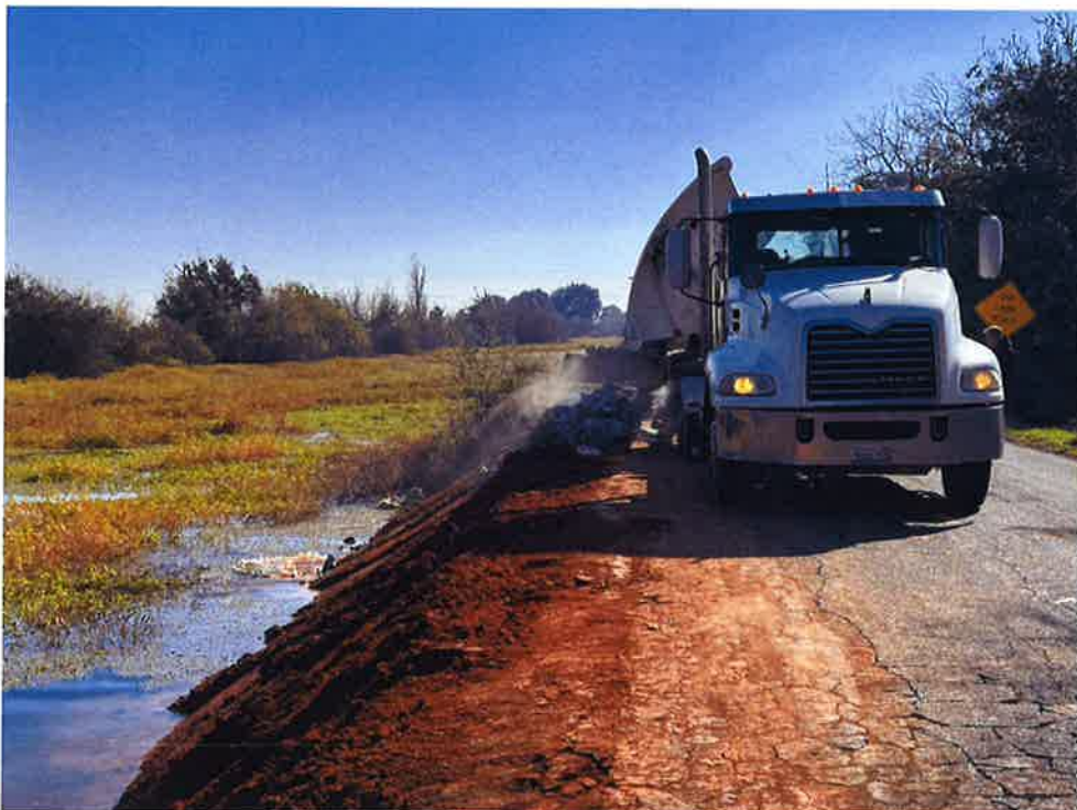
Placement of 18" minus riprap on the waterside levee slope at the western site of repair.
