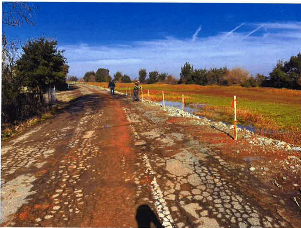
Temporary guard rail placed after completion of the repair (western site of repair).
