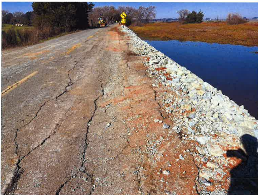
Final placement of riprap and prior to sweeping of Twitchell Island Road (western site of repair).
