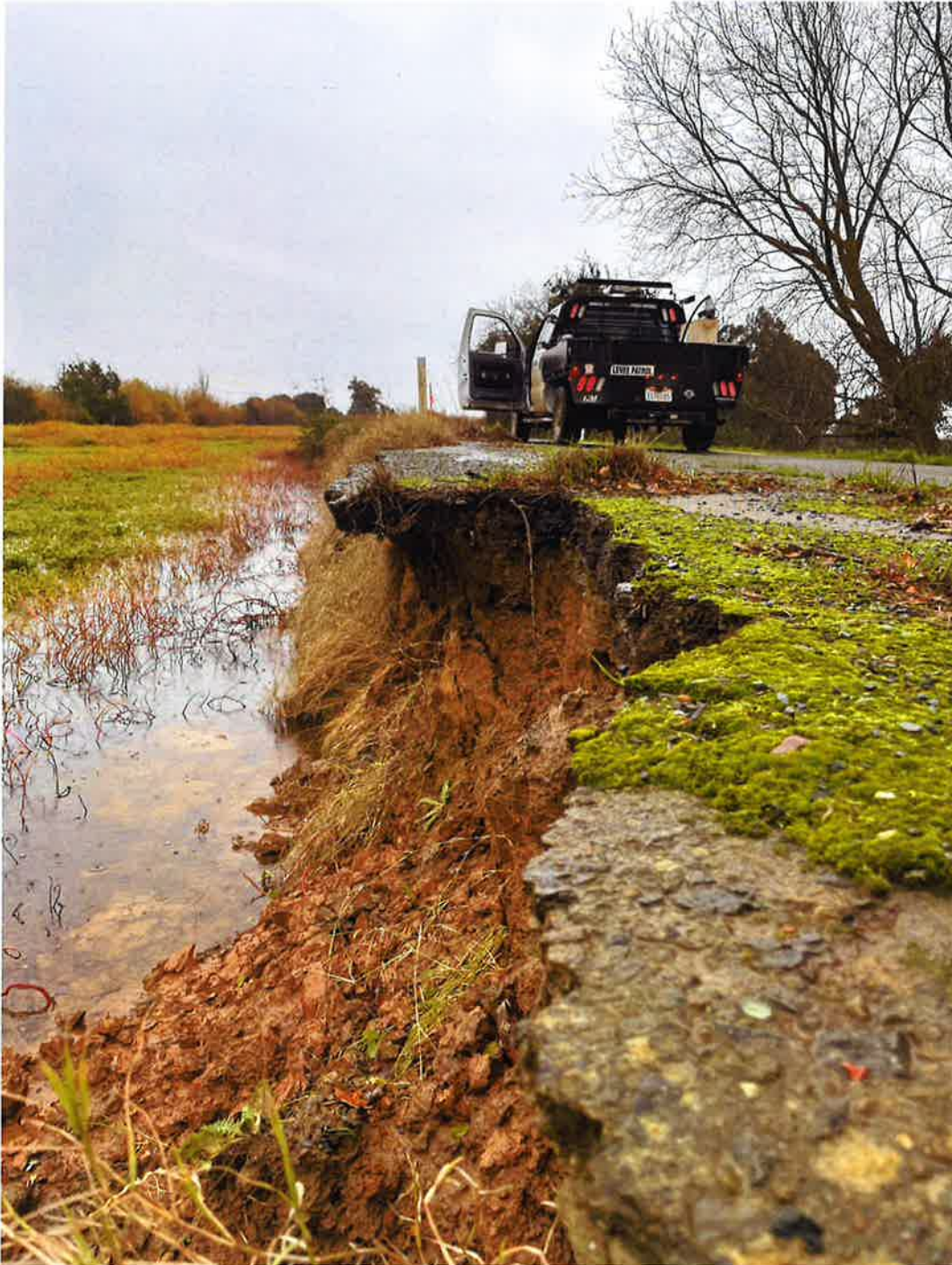
Following the sloughing of the waterside levee slope along Twitchell Island Road, the pavement cantilevers over the slough (photo taken near sta. 190+00 before initiation of emergency work).
